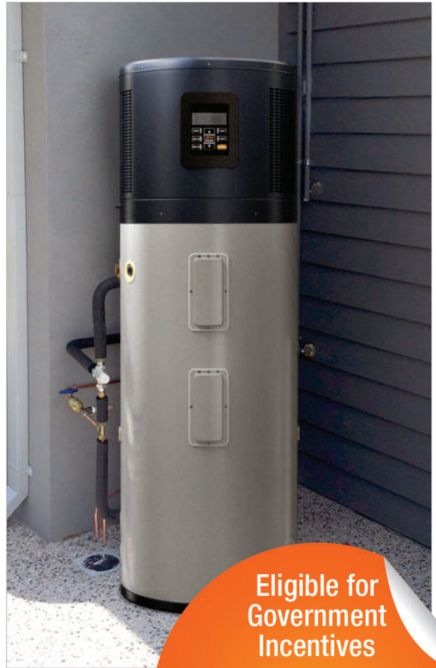
280L Installed Unit
